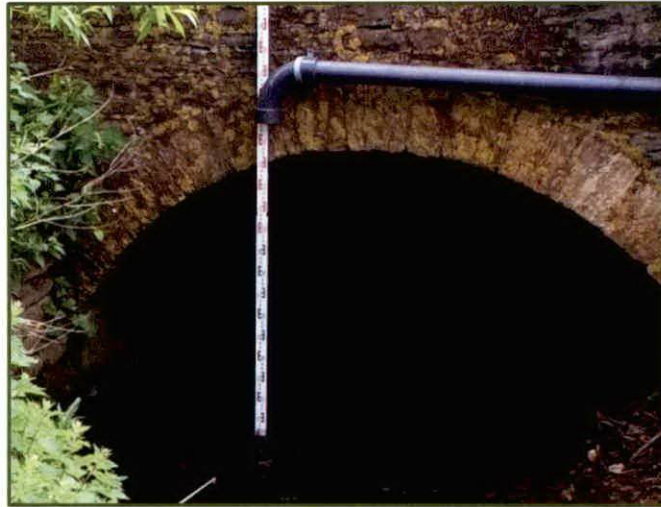
Figure 5.2. Road Bridge Orifice
